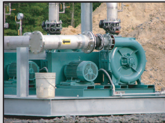
Landfill gas blowers create a vacuum to draw the landfill gas from the landfill wells.
