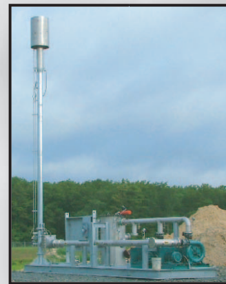
Landfill gas flare during the day.
