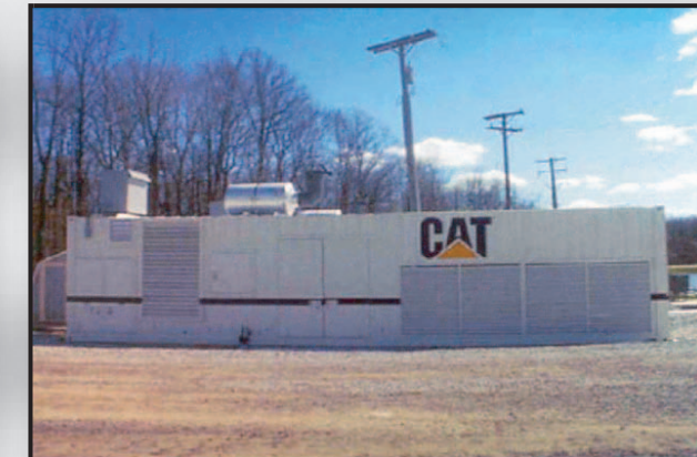
The engine/generator uses the landfill's condensed and cooled landfill gas to power the generator.
